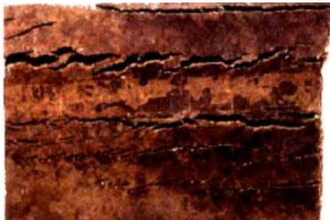
Figure I.11 : Fissures de CSC.
