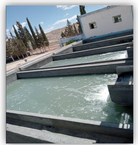
Figure II-9 : station de filtration
