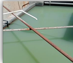
Figure II-3 : Injection de chlore
