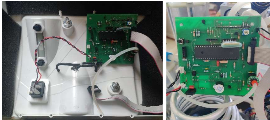
Figure 3.45: Control and display board inside POC.
