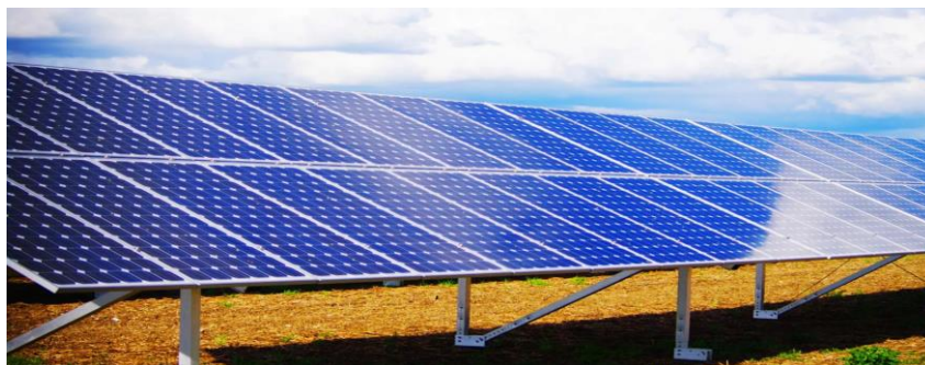
Figure 1:Solar power panels
