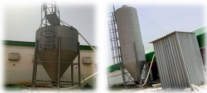
Figure 19: Silos de stockage – B1 et B2 (photo originale,2025)
